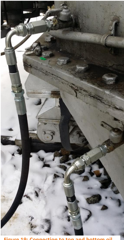
Figure 19: Connection to top and bottom oil
