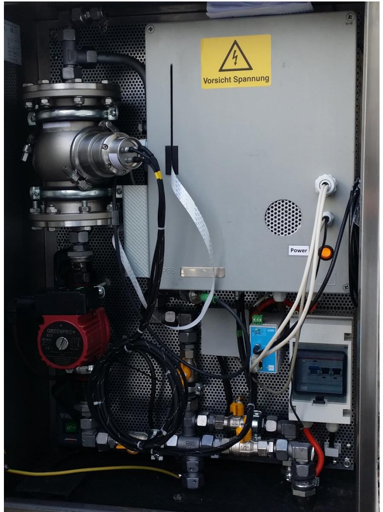
Figure 6: interior of the TranSCoM Online
