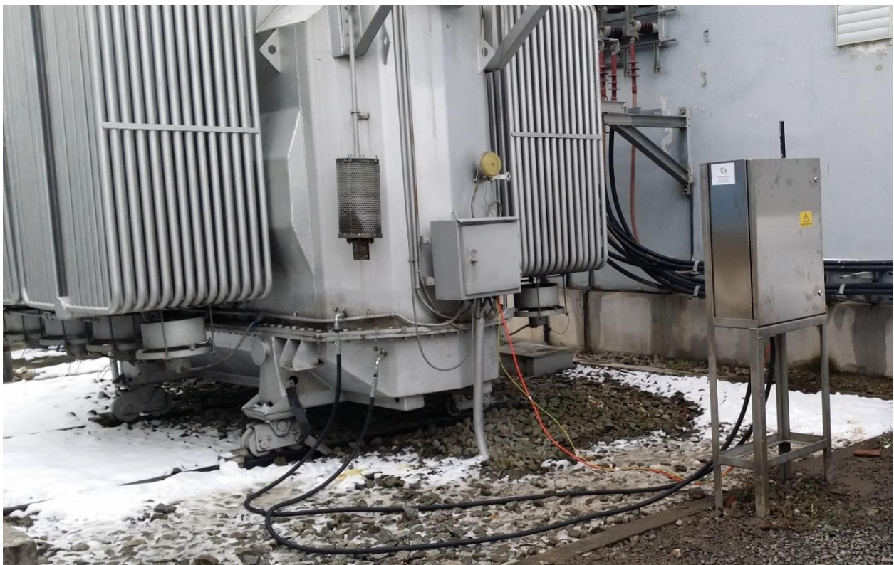
Figure 18: TranSCoM Online mounted on a stand and connected to the transformer
