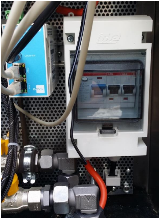
Figure 9: breaker and GPRS modem
